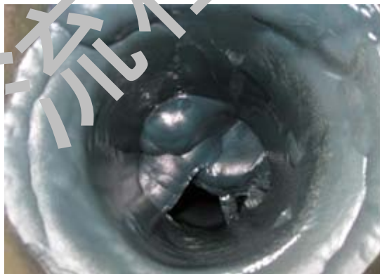
1.5" Thick Deposit on Carbon Steel 1.5英寸厚的积垢在碳钢上
